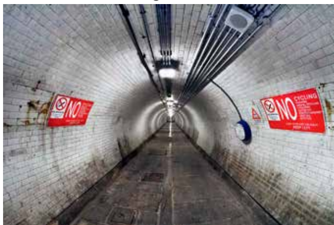
After years of use the white ceramic tiles are looking very dirty in this view looking south before the tunnel was refurbished in 2011. Photo from Hartwell Photography
